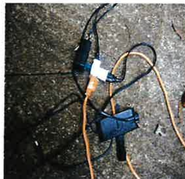
#5 Temporary electrical boxes, lights, cords, and power strips subject to the weather MUST be listed for outdoor use
